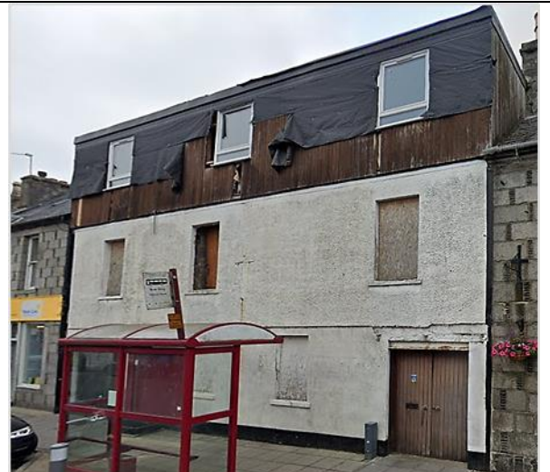
The poor condition of the Grapes Hotel on Victoria Street
