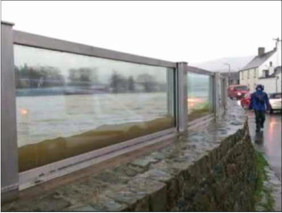
PHOTO 3: EXAMPLE OF EXISTING STONE WALL WITH TOP MOUNTED GLASS AND STAINLESS STEEL FLOOD PROTECTION PANELS (RIVER GREAT, KESWICK)
